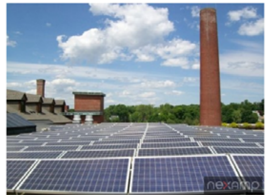
67 kW Solar PV System North Andover, MA
